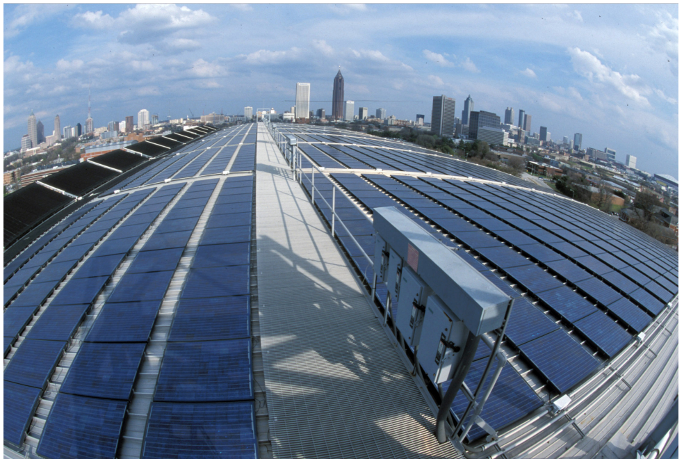
Georgia Tech Solar Panels Photo Credit. Georgia Tech Research Institute / Wikimedia Commons
