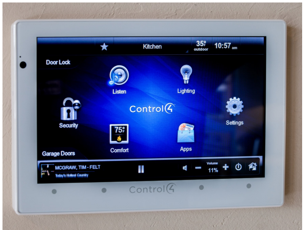
Energy Monitoring System Photo Credit. U.S. Department of Energy
