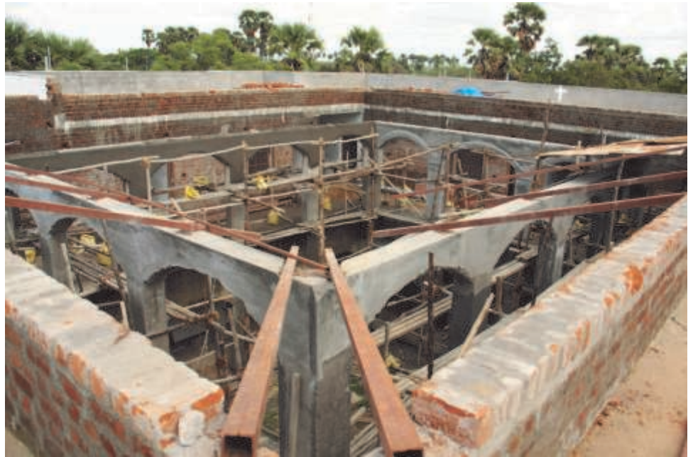
Almost finished. This is the new orphanage (phase 1) at the end of November. It should be ready for occupation early next year (the ready money is on sometime near Easter). Sr. Maria Immaculata, as the site manager of the site manager, will no doubt sing Te Deums from the rooftop when it is all over ...until the next phase begins, that is.
