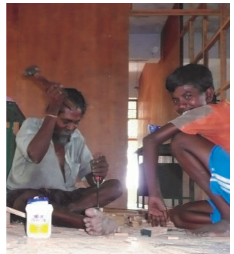
Local carpenters using traditional methods and traditional materials (the batons were made of teak!).
