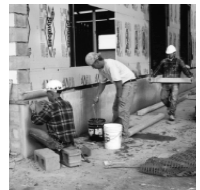
Masons install the limestone base around the perimeter of the building. The rest of the exterior wall surface will be faced in brick.
