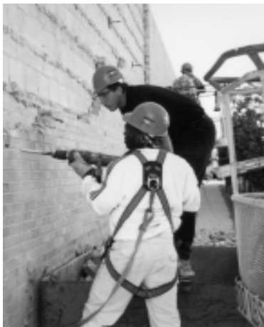
Old brick is removed as the former department store undergoes transformation to the new Mackinac Center headquarters.
