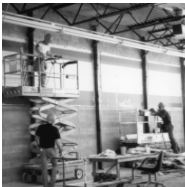
Workers use construction material donated in part by Haddix Lumber of Midland.
