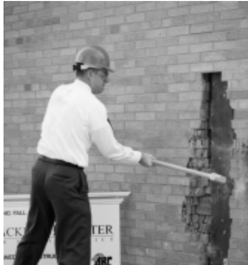
Buckeye Institute President Richard Leonardi helps the Mackinac Center symbolically break ground on its $2.4 million new headquarters project (see page 7). The headquarters is being built on the site of a former department store.
