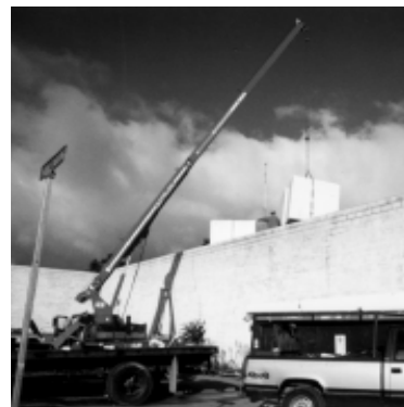
Over $20,000 worth of Styrofoam insulation, manufactured and donated by The Dow Chemical Company, is hoisted onto the roof.
