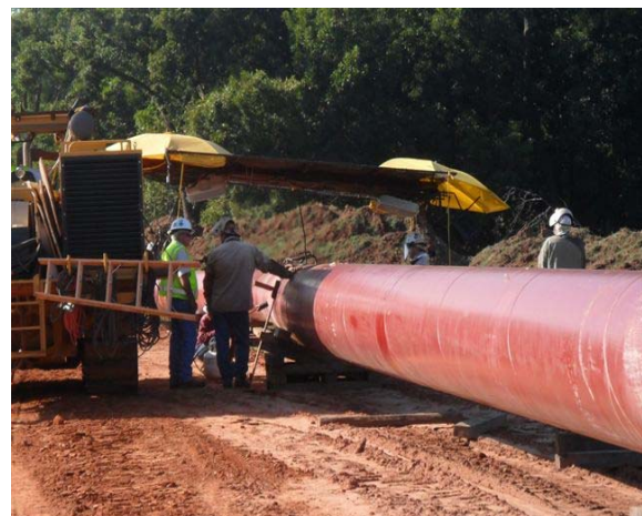
Figure ES-2 36-Inch-Diameter Crude Oil Pipe
