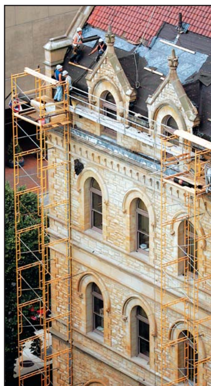
Construction workers install a new roof on the building owned by the law firm of Bricker & Eckler, which has spent a lot of money to maintain it.
